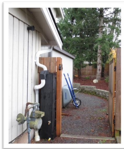
Rainwater harvesting system installed to water new native plants.
